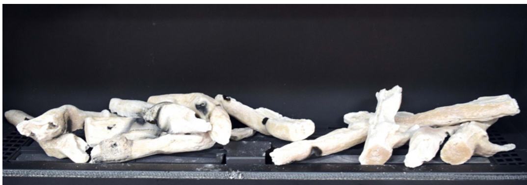
Incorrect Media Installation
