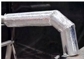
Bends where practical should be insulated, by cutting the insulation into segments and taping together.
